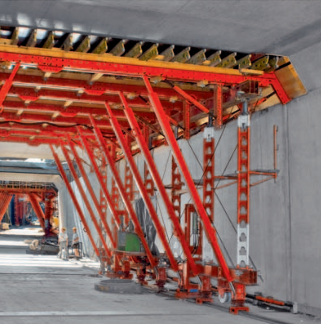
HD 200 heavy-duty props installed in the trailing slab formwork carriage accommodate the loads of this road tunnel constructed using the separate casting method.
