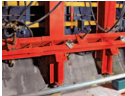
The experience gained from brace frame anchoring can also be used in the 2nd cycle.
