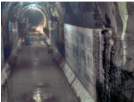
Best concrete results from the 2nd cycle (wall area) form the exit for the arched formwork carriage.
