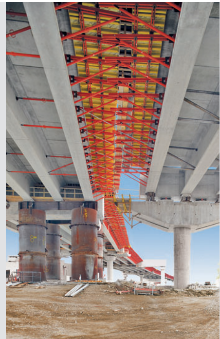
Semi-prefabricated concrete component construction method Golden Ears Bridge, Canada Prefabricated concrete girders with in-situ concrete slabs.
