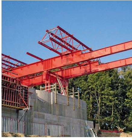
Assembly of the sub-assemblies in a position behind the abutment is the rule regarding initial assembly. At the same time, passing the abutment wall is a factor that must be taken into consideration.
