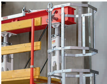
Ladders with safety cages, which are attached to the prop chords, guarantee safe access.
