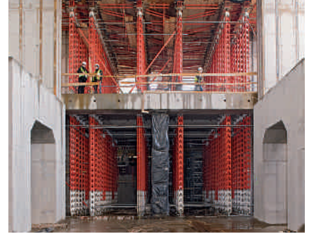
Transferring high loads with low space requirements – making full use of the advantages of the HD 200 Heavy-Duty Prop for the construction of a power plant.
