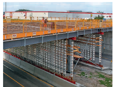
HD 200 as main beam section for the building of a road crossing using a steel composite construction method.
