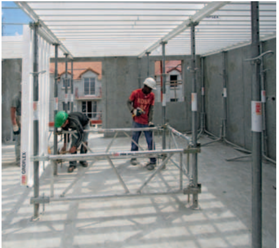
The PERI Ergo tripod and the PERI PRK frame are used as assembly aids.
