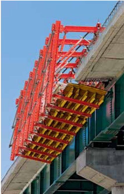
With the diagonal spindles, all inclinations and heights for the cantilever formwork could be easily adjusted.
