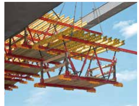
The project-specific solution with lightweight raised formwork units ensured fast and simple moving to the next concreting section with the crane.
