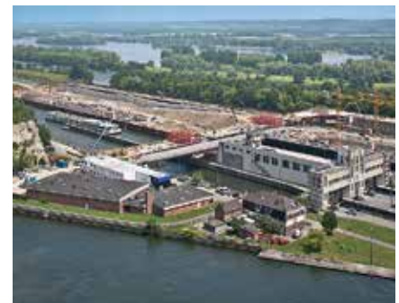
The expansion of the Lanaye lock facility required construction of a new 200-m-long road bridge complete with two 90° bends on the river bank areas.
