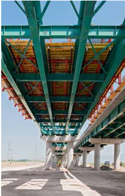
The two parallel superstructures of the the 22-field bridge were built using the steel composite construction method.
