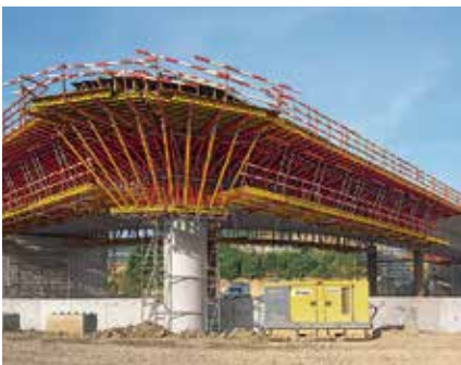
In the complex area featuring the extremely narrow outer radius, the concentrated loads of the radially arranged cantilever brackets were transferred by means of pressure-resistant ties into the existing bridge pier.
