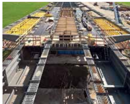
In spite of the geometric changes found in the superstructure, only two standard raised formwork units were used which resulted in a very high degree of material utilisation.
