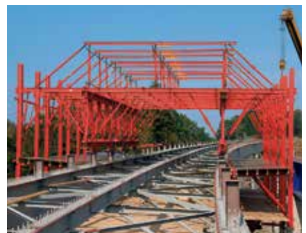
Striking can take place either from the concreting level or the finishing platform.
