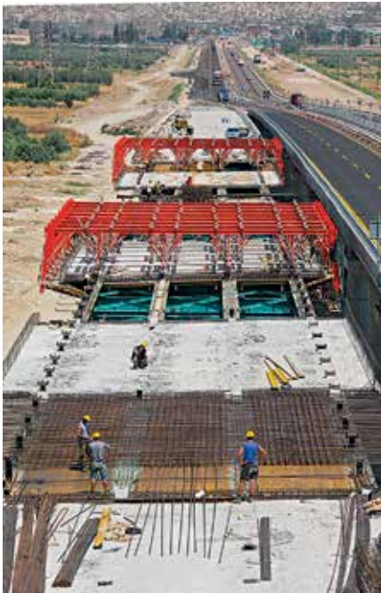
With the help of the two formwork carriages and two additional sets of slab formwork in advance, the field and pier concreting cycles of up to 22.50 m were carried out using the so-called back-step method.
