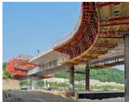
The steel composite bridge was constructed using formwork carriages and cantilever brackets taken from the VARIOKIT product range.
