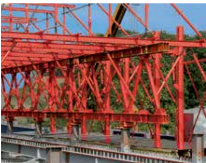
Load transfer takes place via the cross-frames and longitudinal truss on the formwork carriage supports.
