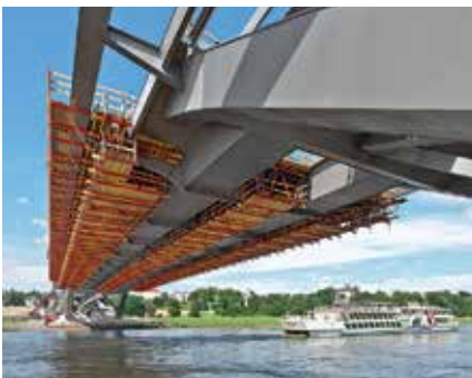
The carriageway of the steel composite bridge was constructed using 21 concreting sections. The raised formwork units were based on rentable system components taken from the VARIOKIT Engineering Construction Kit.
