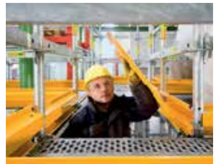
Hatches painted in a yellow signal colour can be opened in a sideways direction. They close automatically which eliminates any source of danger.
