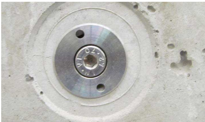
Photo 2 Screw plug "Schraubstopfen MX 15-50 MF-LS" Unexposed face before fire test
