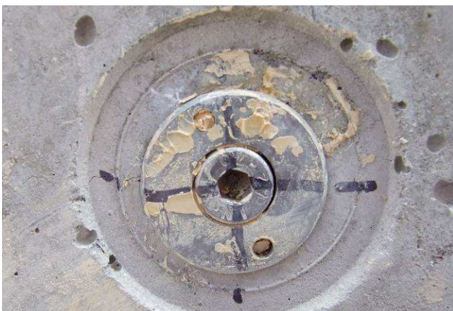
Photo 6 Screw plug "Schraubstopfen MX 15-50 MF-LS" Unexposed face after fire test
