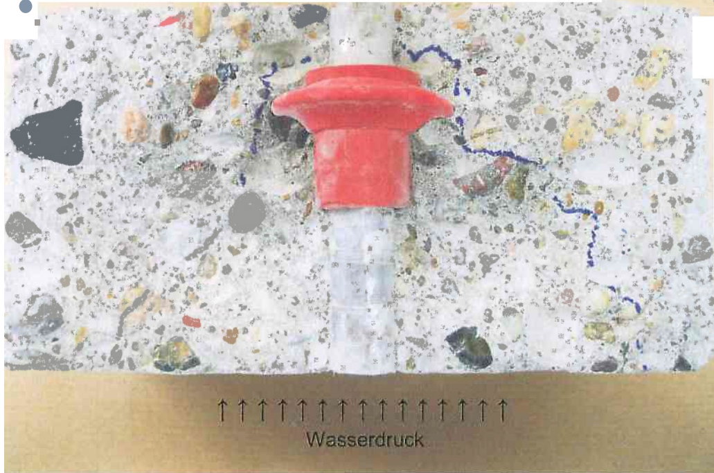
Picture A2: sample 1: tie rod (ripped steel \varnothing = 16 mm)
